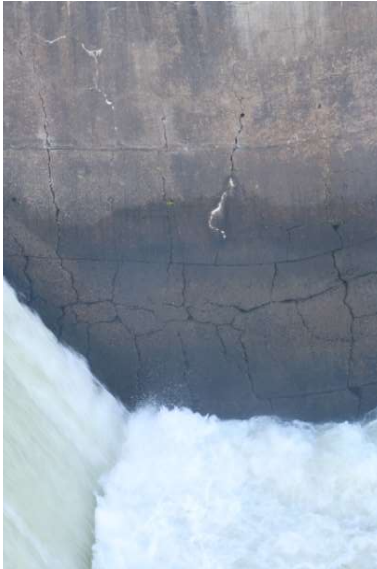
Figure 5: Cracks in NSBLD
