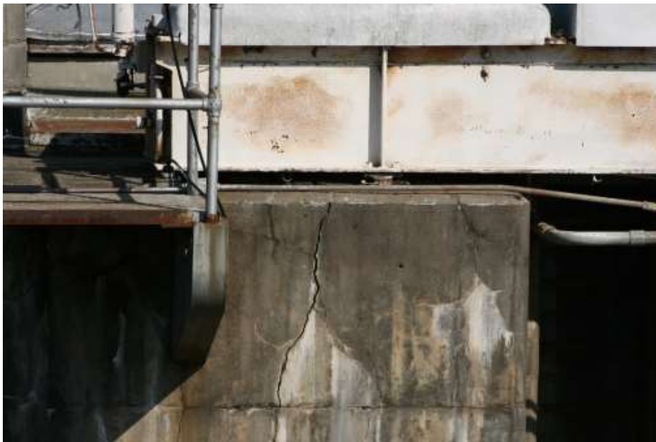
Figure 4: Cracks in NSBLD
